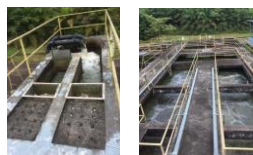
(a) Primary treatment and (b) aeration and sedimentation tank of STP 3 in Universiti Teknologi Malaysia
